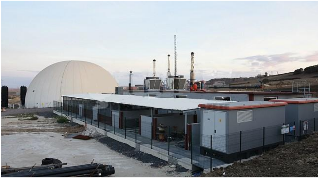
Figure 1. Panab Corlu Biogas Plant
