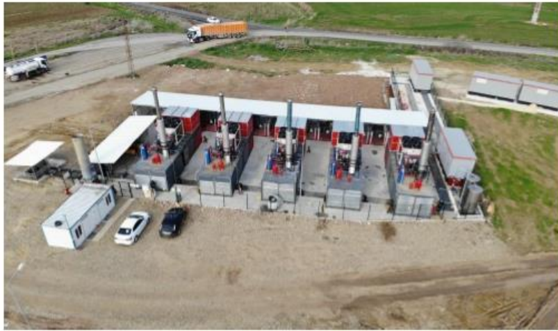
Figure 1. Panab Tekirdag Biogas Plant
